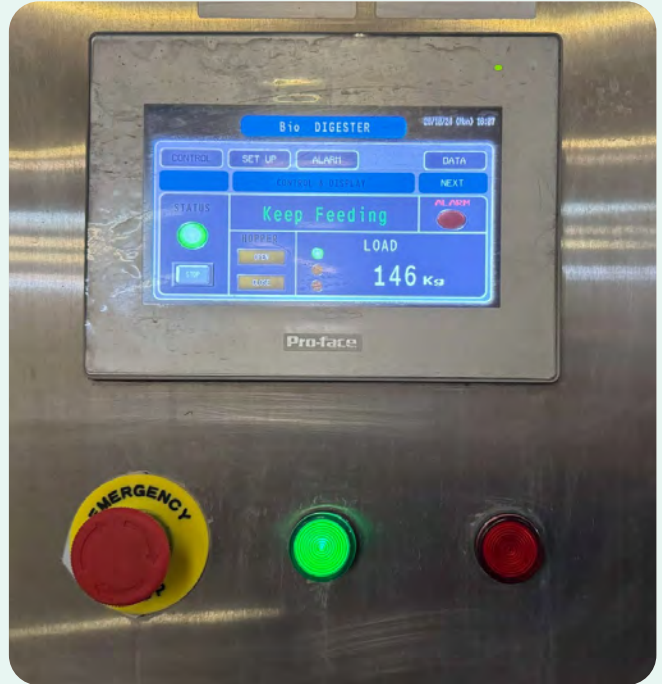
▲ The panel on the food waste treatment system showing the weight of the food waste contained.
