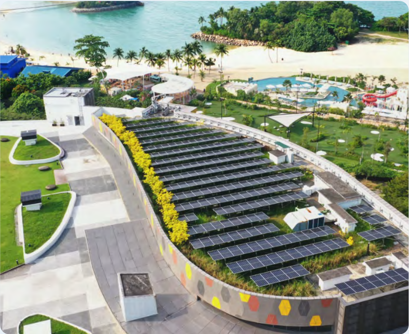
▲ Solar panels installed on the roof top of Palawan Kidz City, amongst 45 other locations across Sentosa and Lazarus Island.
