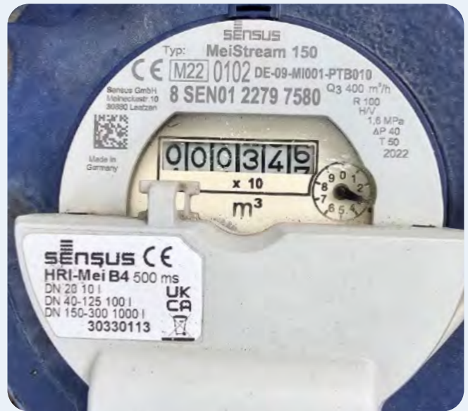
Smart water meter at Heritage Conservation Centre. ▶
