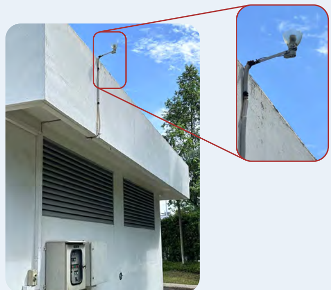
A rainfall sensor-controlled drip irrigation system at MOM Services Centre. ▶
